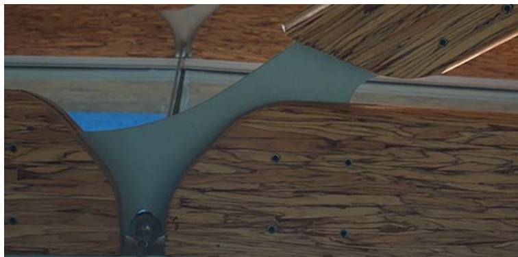
Figure 6: This detail shows the connection of the support arm and muntins to the aluminum plate and the intersection of the support cable with the aluminum plate
